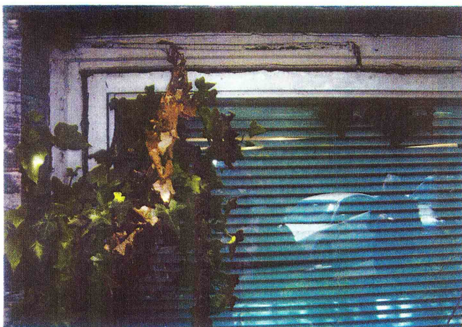
Replacing sash while ignoring the primary sources of infiltration can have detrimental and costly results.
