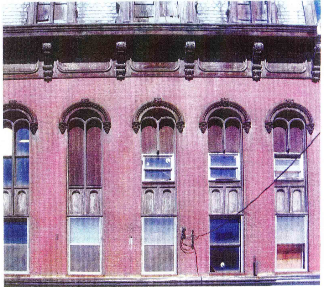
The damage wrought by replacement windows is self-evident and increasingly pervasive. All photos: © Walter Sedovic Architects
