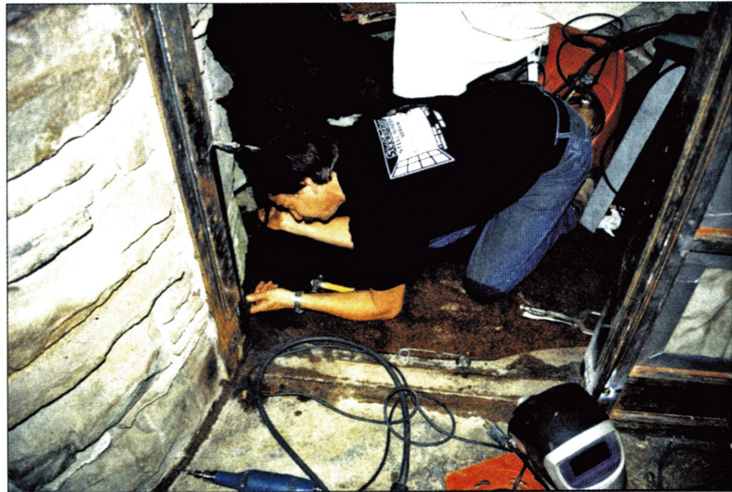
Bobby Seekircher restores a door frame, an effort that required three ten-hour days.
