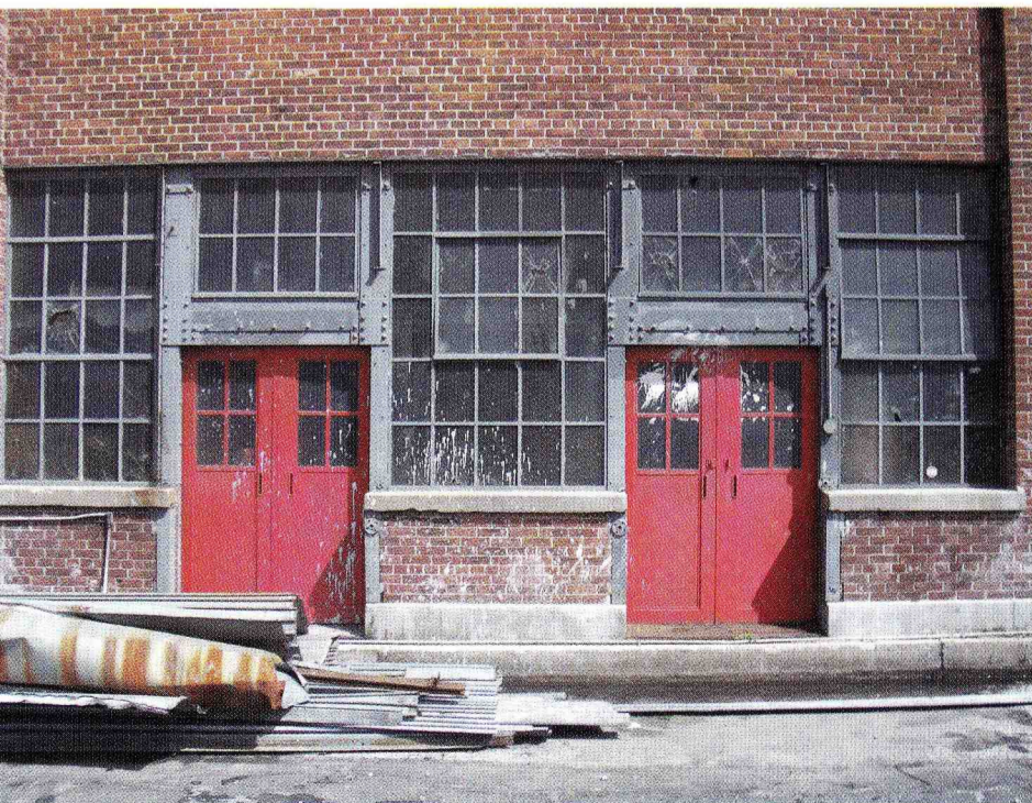
Many of the original window frames were misaligned or missing hardware or glass, resulting in substantial thermal loss and making the building look unattractive.
