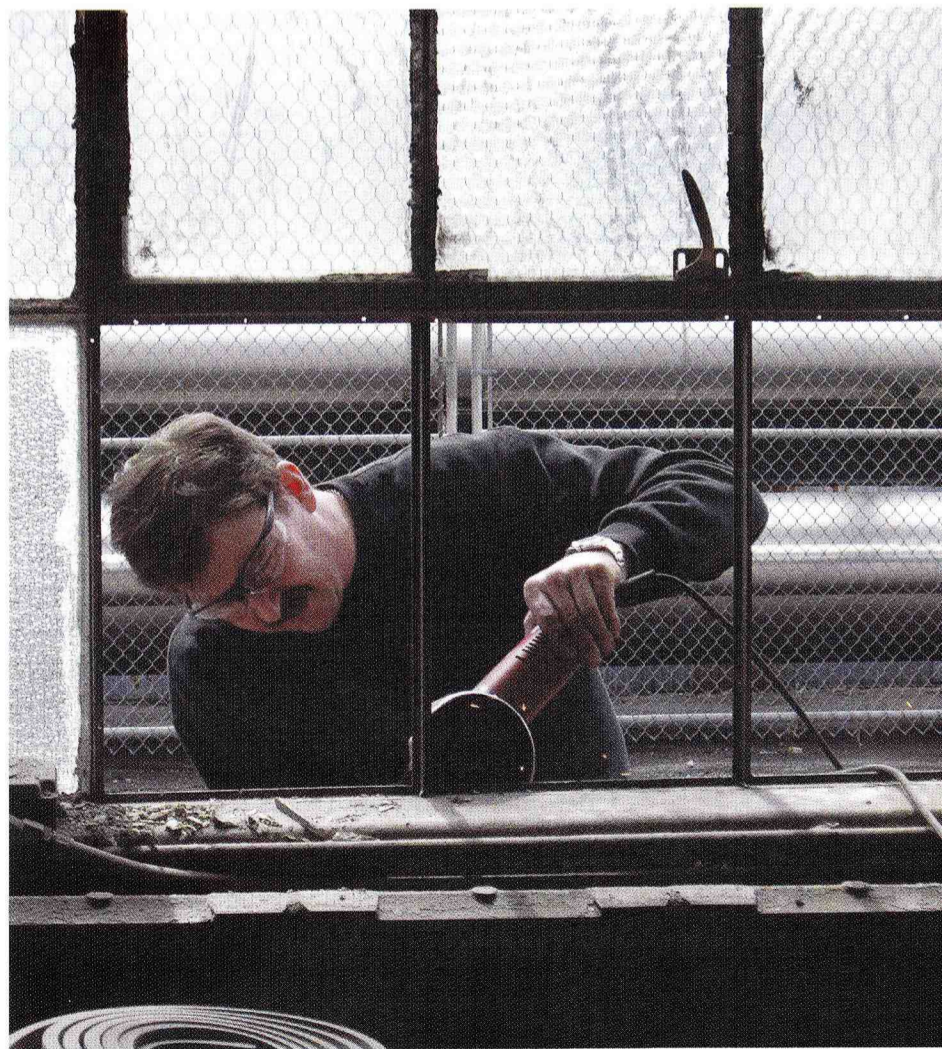
John Seekircher's team, which included his brother Robert (pictured), carried out the restoration in less than eight weeks, replacing more than 1,300 panes of glass and repairing and replacing missing steel and hardware.
